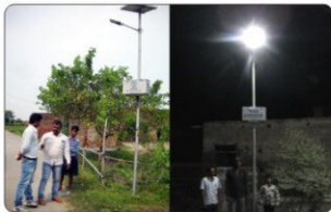
LED based Street Lighting Systems
